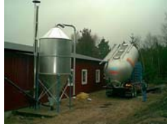
European Installation, 2005 Wood Pellet Delivery
