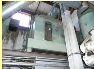
Pellets entering counter-flow Cooling Chamber
